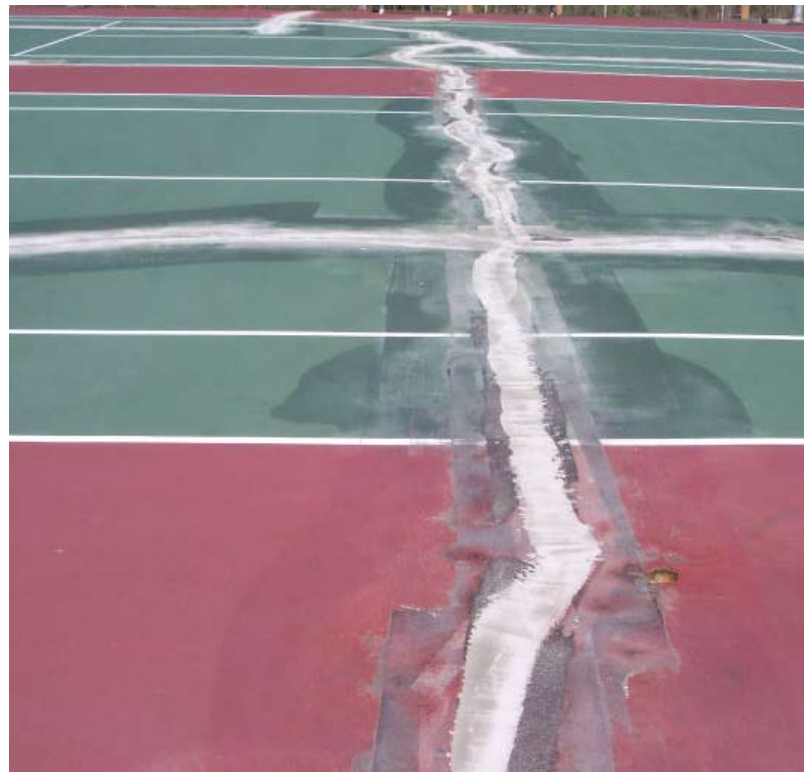
Properly filled crack. Routed and filled from bottom up, then buffed smooth.
