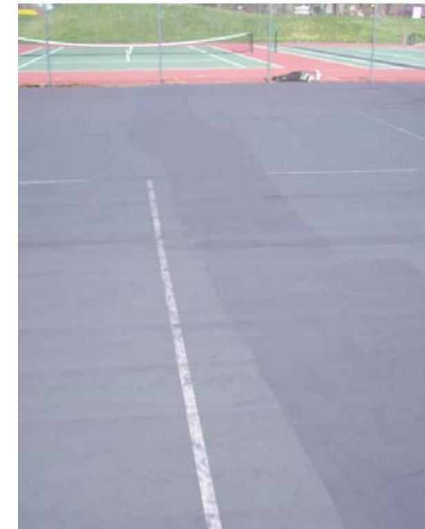
Repairs are coated with acrylic with sand 2-3 time before first coat of resurfacer to entire court. This hides the repair.
