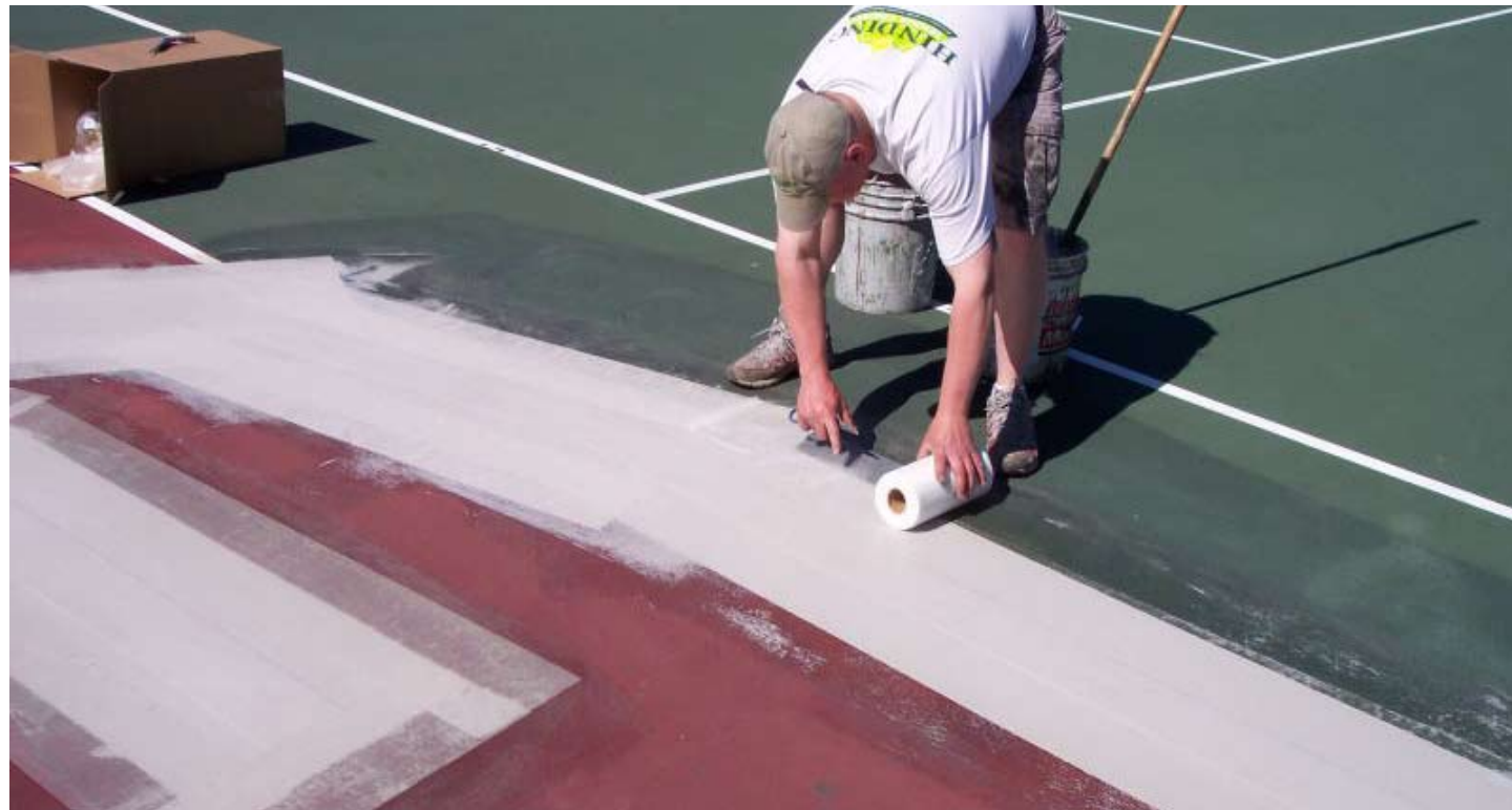
Cutting bonding where crack changes direction, then coating bonding edge with acrylic, no sand.
