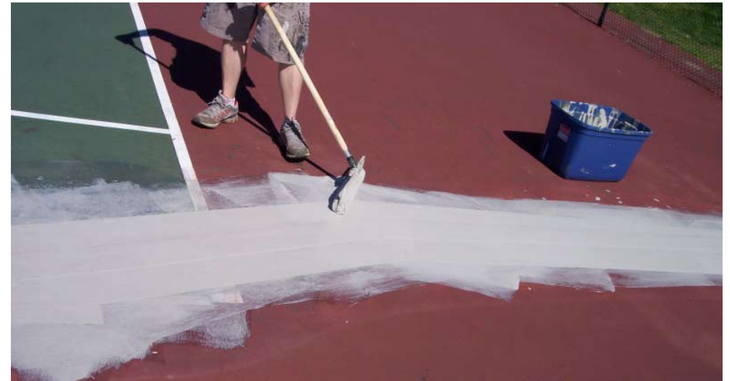
Coating stress matt (fabric) and rolling smooth to ensure no wrinkles or air bubbles.
