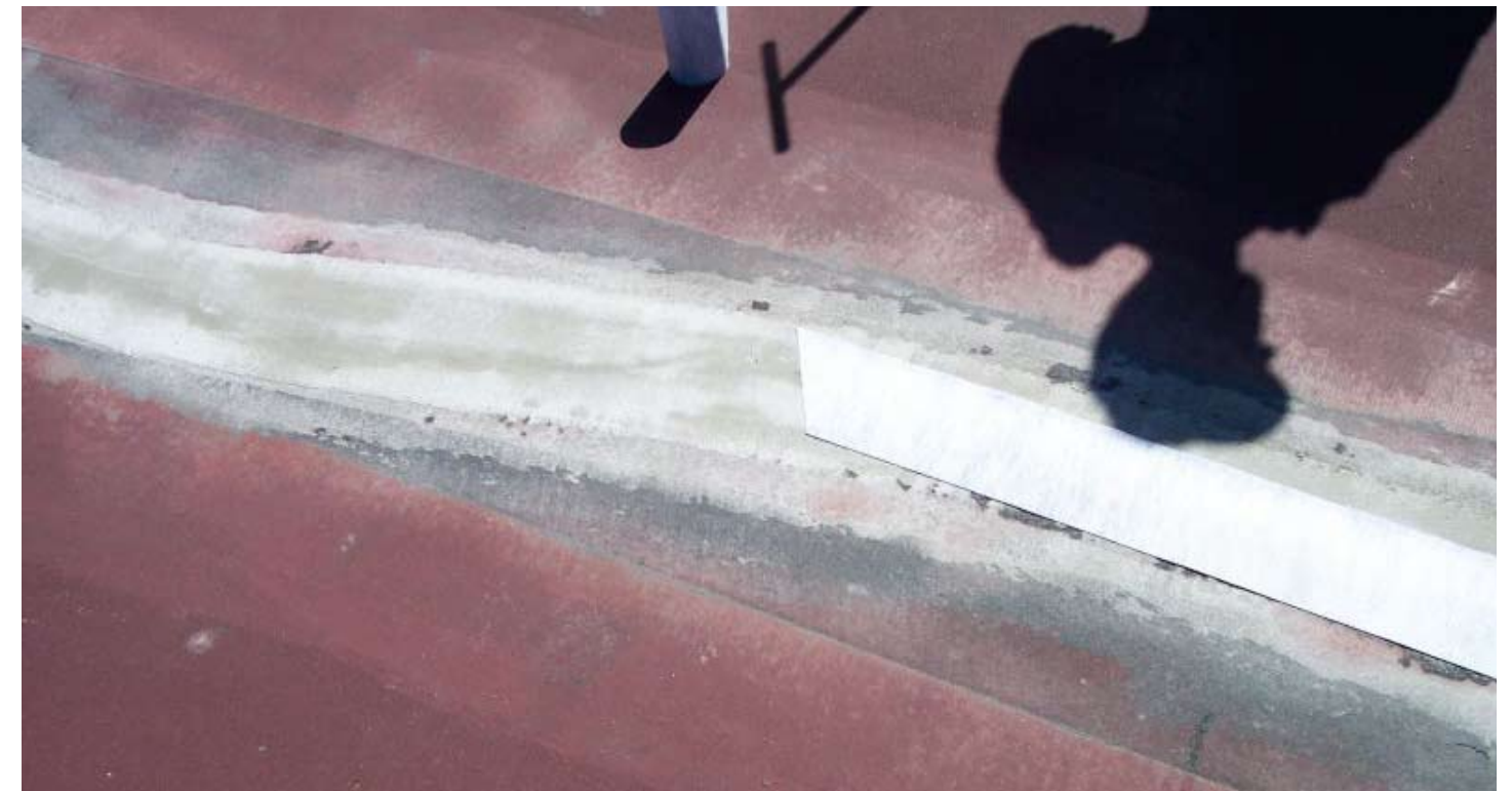
Cutting the tape to match changing direction of crack.
